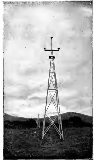
FIG. 2.—ONE OF THE TRANSMISSION LINE TOWERS.
